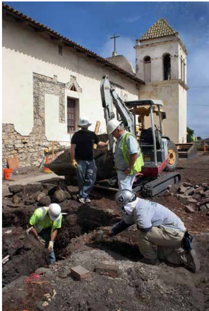
Figure 3. In order to mitigate against the continued deterioration of the shale and mudstone due to water intrusion and salt erosion, the Royal Presidio Conservation Project of the Diocese of Monterey undertook the large-scale installation of a French drain system. In order to see through this process, fourteen 22-foot to 25-foot long and 18-inch wide trenches were excavated to bedrock along the entirety of the perimeter of the Royal Presidio Chapel (aka: San Carlos Cathedral). Photo © Rubén G. Mendoza, 2007.
