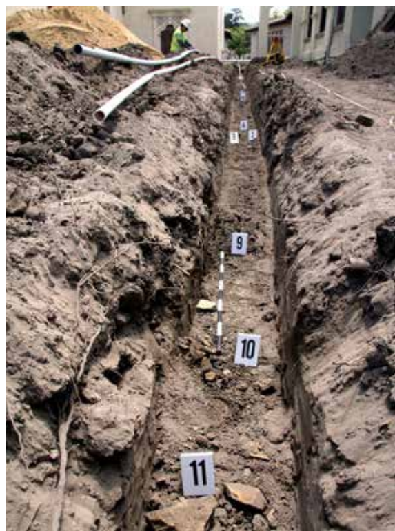
Figure 6. The one-day trenching operation undertaken in the area immediately to the west of the Chapel of 1794 (aka: San Carlos Cathedral) made use of forensic or crime scene evidence markers on an ongoing basis so as to demarcate subsurface architectural features encountered during the course of excavation. The evidence markers in this instance serve to delineate the south (Marker 6) and north (Marker 10) exterior faces of the Missionary's Quarters of 1770. See Figure 7 field map, below. Photo © Rubén G. Mendoza, 2008.
